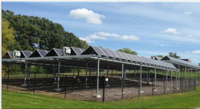
Maplewood City Hall Ground Mounted Solar Arrays
