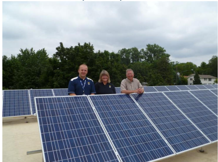
Solar array on the Eden Prairie Community Center. Photo courtesy of the City of Eden Prairie
