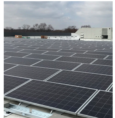
Municipal paneles solares
