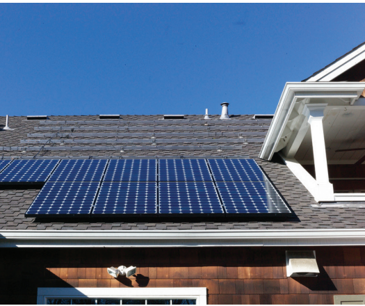
"First ten panels on the roof!" by Jon Callas is licensed under CC BY 2.0
