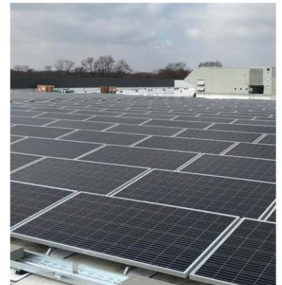
Municipal Solar Panels
